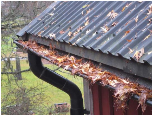
Figure 2. Nuisance from leaves in the roof gutter (Sewer, 2022)
