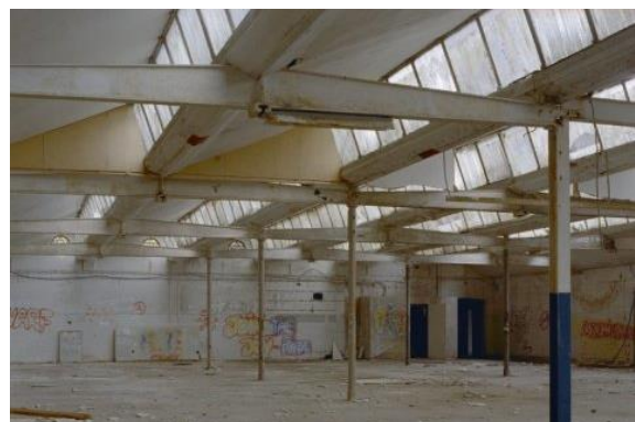
Figure 2.5. [Interior of the former Herman Driessen steam weaving mill in Aalten, built in 1893]. Adapted from Cultural Heritage Agency website, by IJ. Heins, 2002, retrieved from https://beeldbank.cultureelerfgoed.nl/ Licensed under a Creative Commons Attribution-ShareAlike 3.0 Generic license, http://creativecommons.org/licenses/by-sa/3.0/
